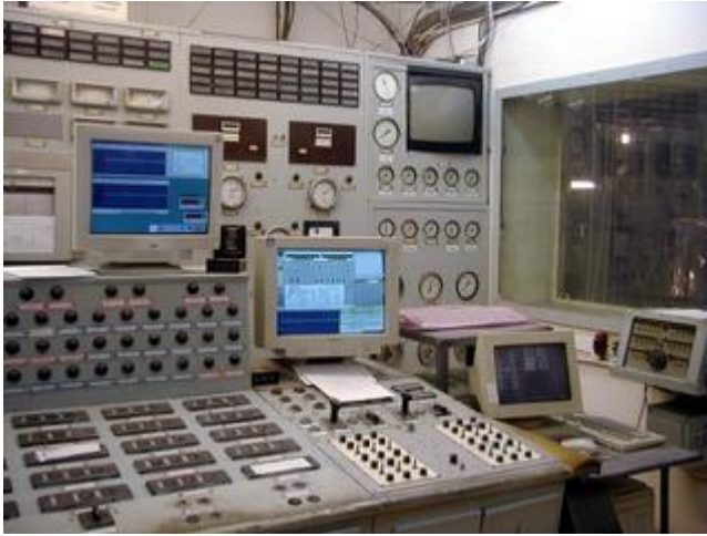
Figure 2. DASOP shows operational and safety information in real time.
