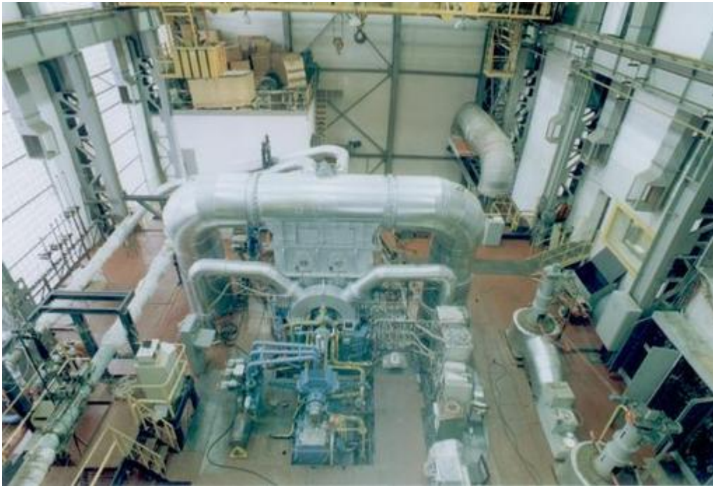
Figure 1. The turbine under test is in the center, surrounded by steam pipes and test equipment.
